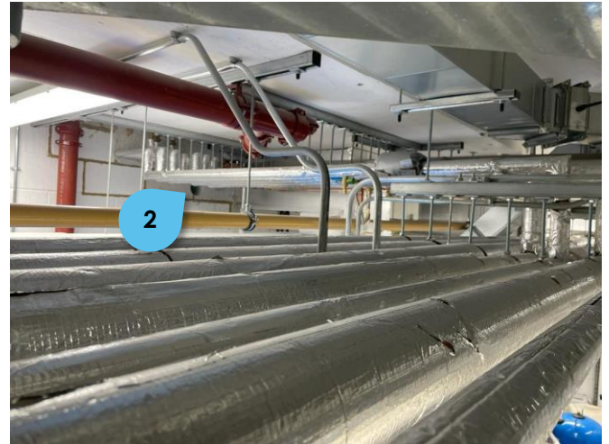
MAIN PLANT ROOM (B)
